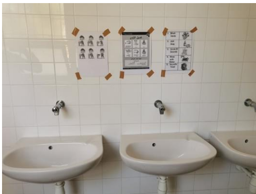
Washroom in the Guarded Refugee Reception Centre with information material on proper hand washing
